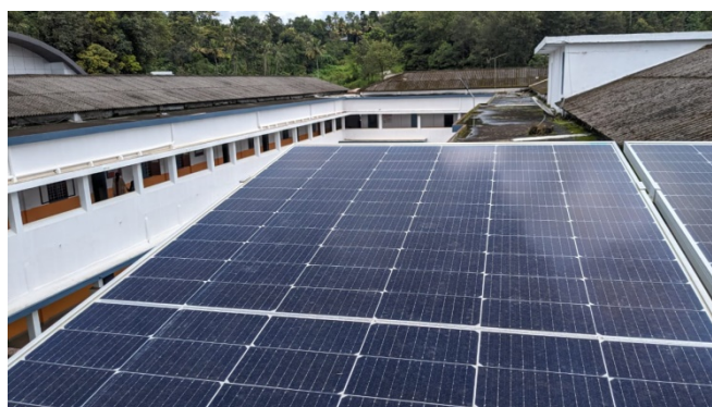
10kWp Solar Power plant
